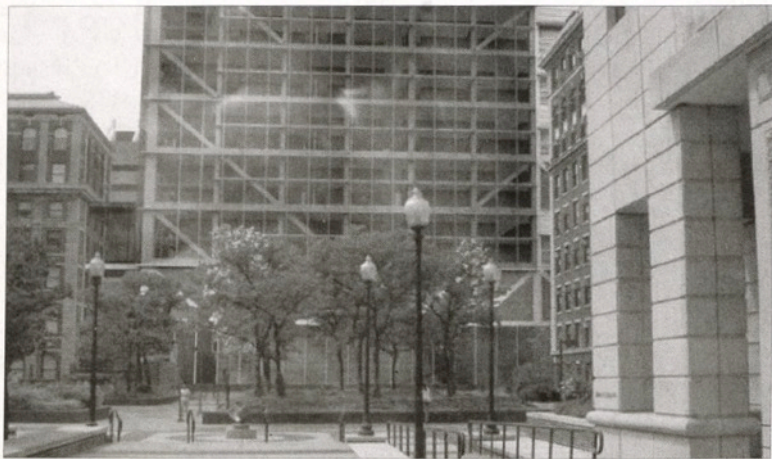
GOING UP | The northwest corner project will provide the University with a new research building, seen here, as well as bridges integrating existing chemistry facilities with the science and engineering terraces.
