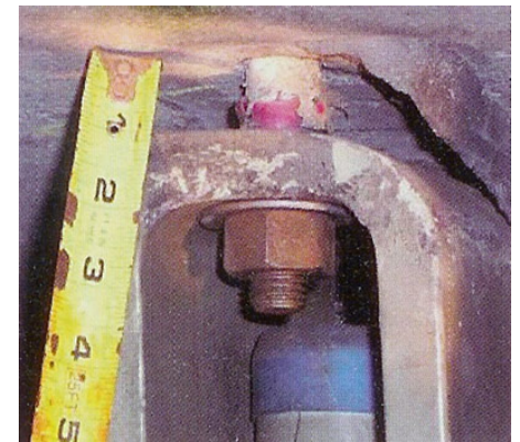
Failing anchor bolt
